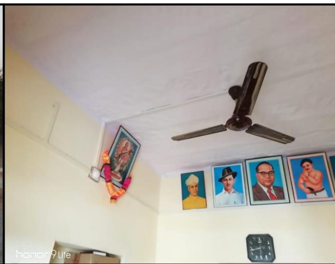
Electrical appliances running on solar power
