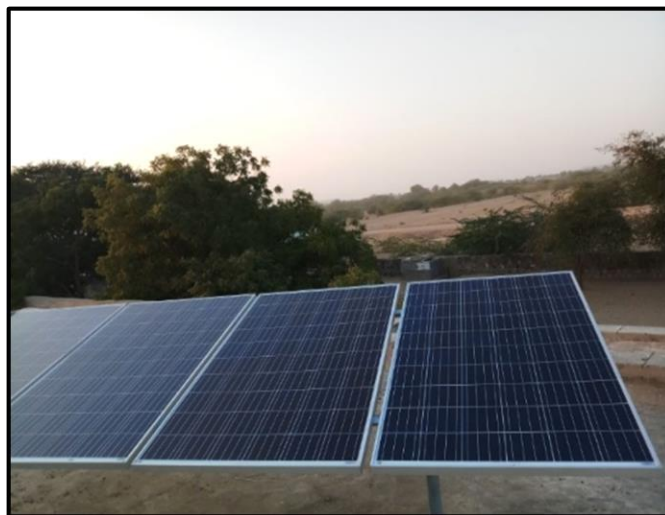
Solar panel mounted in Adarsh schools
